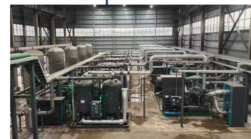
Provision of EPC services for a class 1 energy-efficient air compressor station including various aftertreatment equipment.
